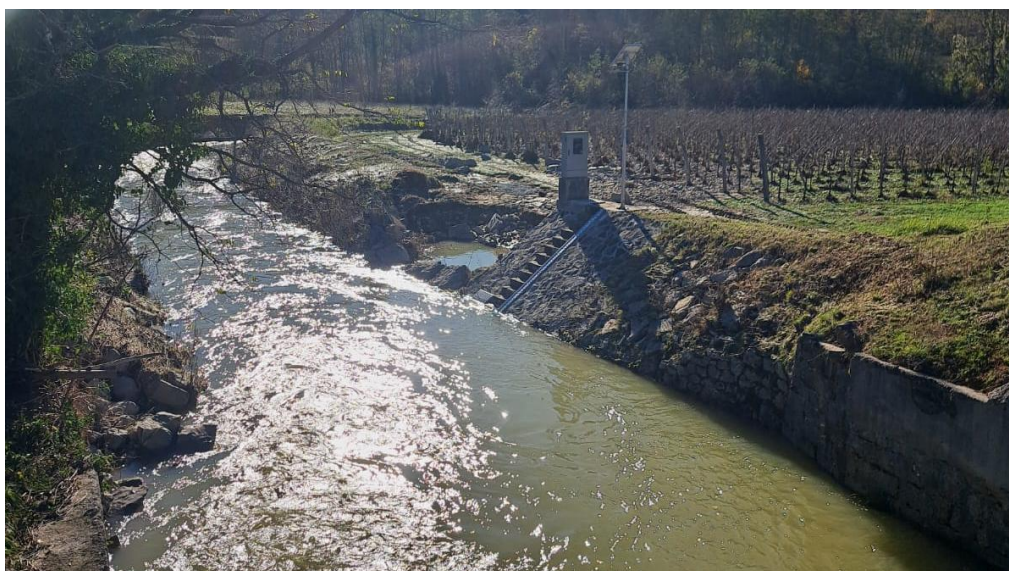
Slika 3. Ob poplavih poškodovan desni breg Kožbanjščka ob vodomerni postaji Neblo, 18. november (foto: arhiv ARSO) Figure 3. The right bank of the Kožbanjšček River near the Neblo gauging station damaged by floods, November 18 (photo: ARSO archive)
